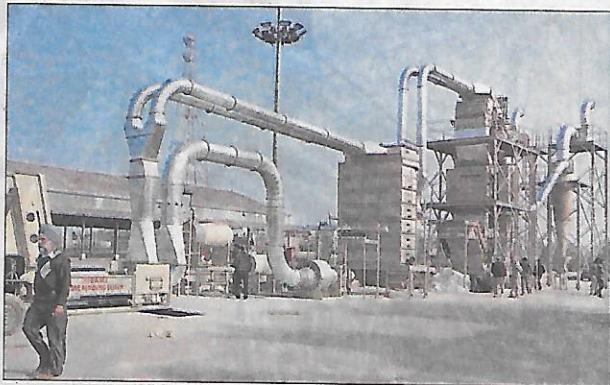
■ The cotton-cleaning and drying plant installed at a cost of ₹1.25 crore in the Malout grain market of Muktsar.
